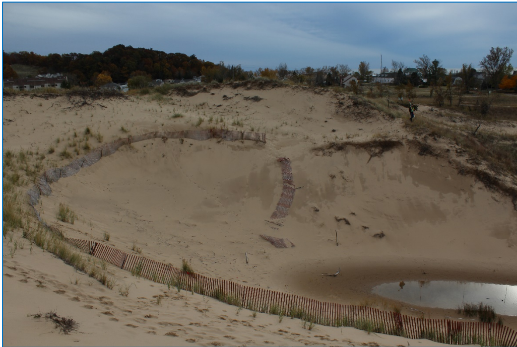
Figure 7. Sand fence wraps around the upper slope of the deflation area. One section (visible in center of photo) has collapsed and is resting on the dune surface.
